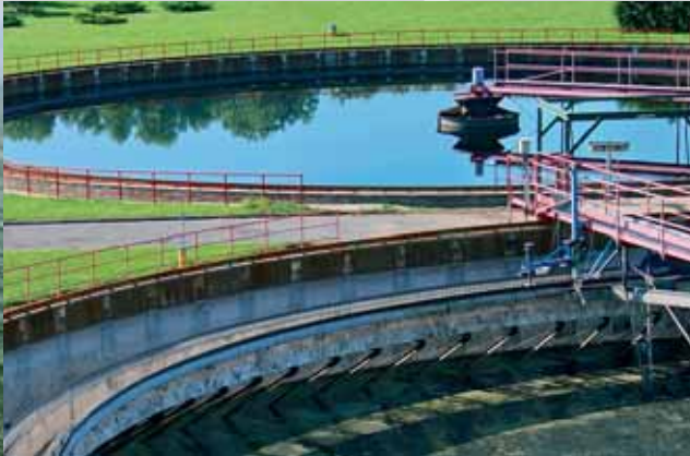
Three VLT® Low Harmonic Drives installed at waste water station ensure compliance with IEEE519.
